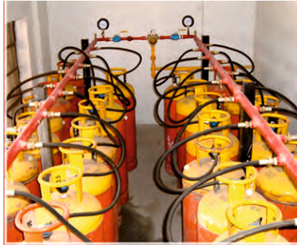
LPG BANK PIPELINE
